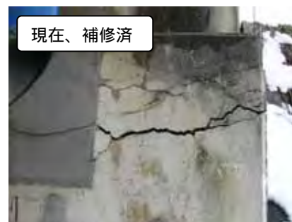
A S R劣化橋梁
