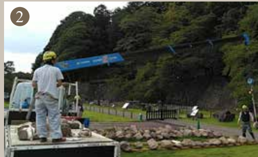
2 We bring stones from the collapsed walls to Imoribori-enchi Park.
