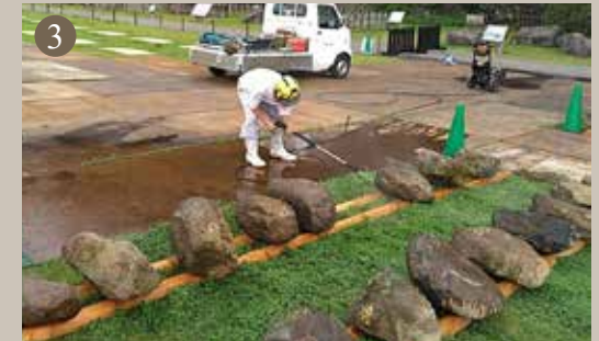
3 We check for cracks and breaks, and wash away any mud stuck to the stones that could cause the walls to collapse or deform.
